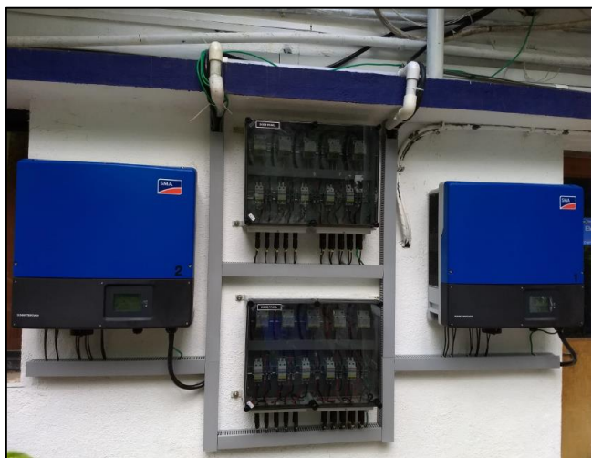
DC junction box and Inverters
