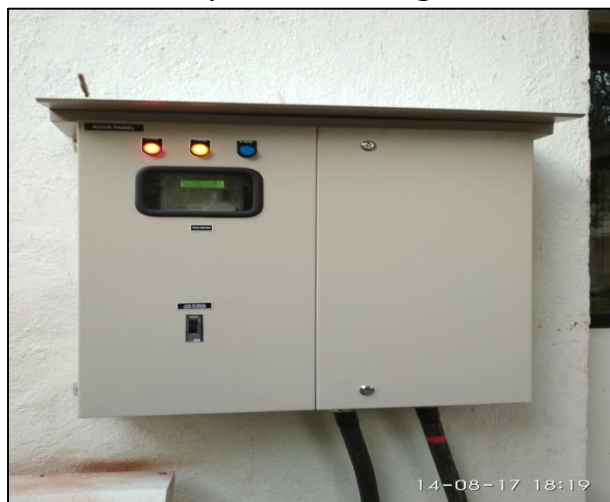
AC distribution box
