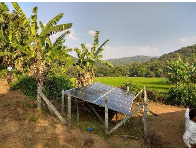
Solar PV Generation
