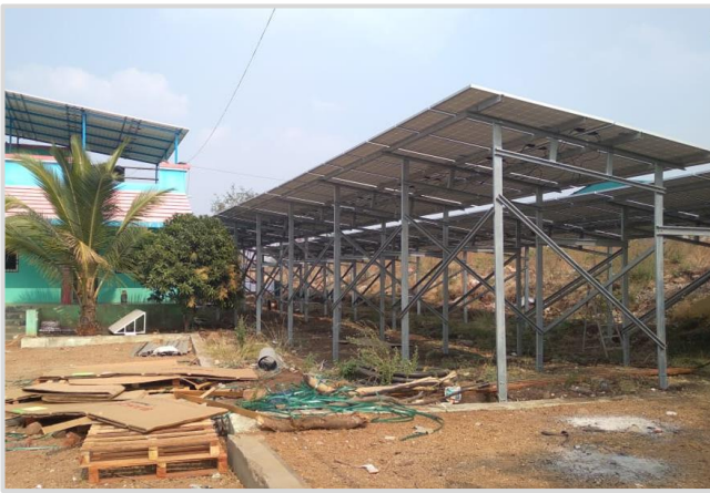
Ground mounted super structure
