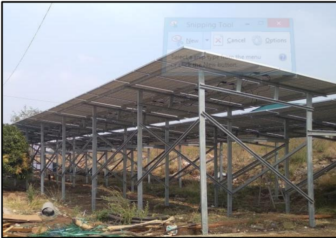
Ground mounted Super structure
