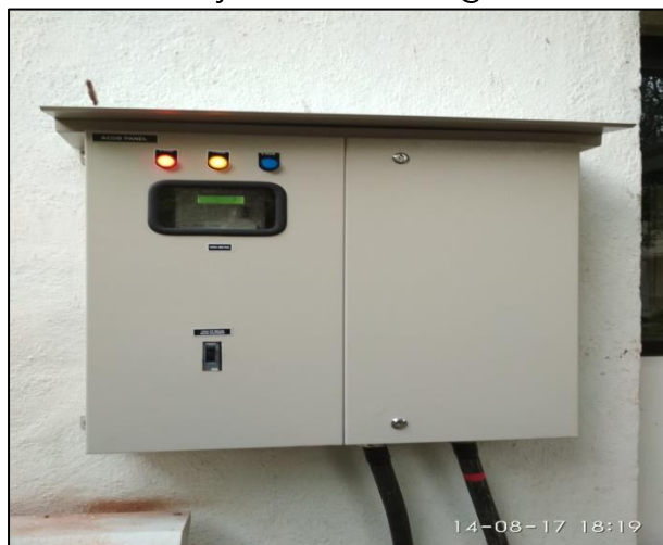
AC distribution box
