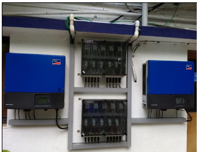
DC junction box and Inverters
