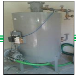
H 2 S Scrubber & Pressure Regulating System
